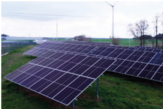
Rys. 2 Farma PV – 0,5 MWp
