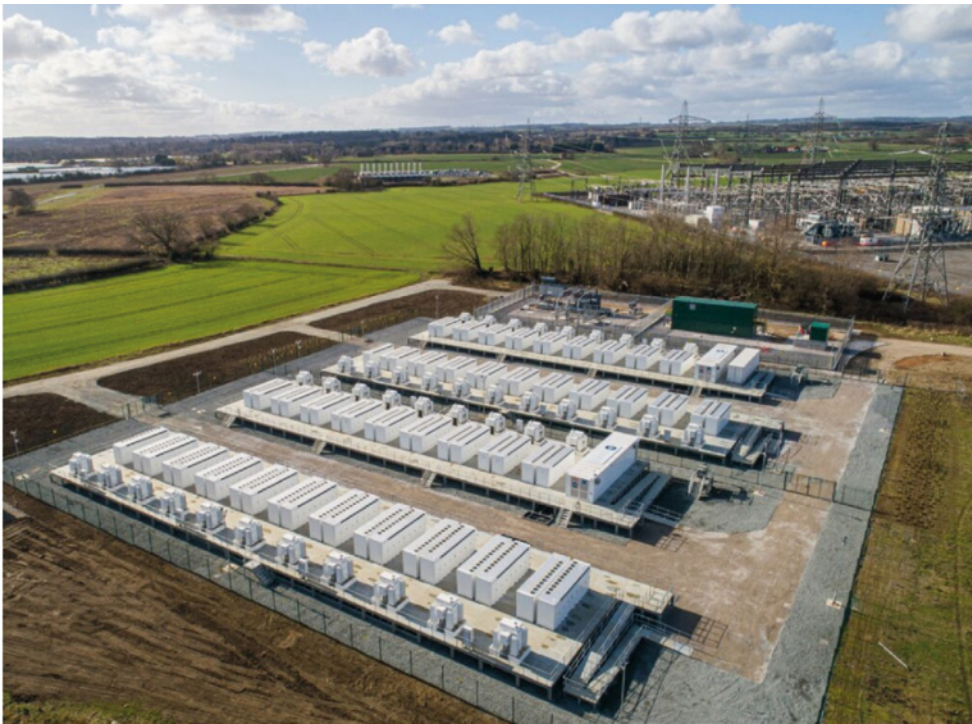
Fig.4. Battery electricity storage Pillwood in Cottingham in UK – Europe's largest battery energy storage system (BESS), MWh [5]
