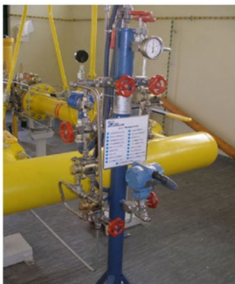
Fig. 8. View of the CRONOS reduction and protection devices and the LC-21 control unit [3].
